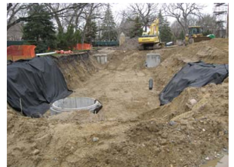
South Storm Retention System
